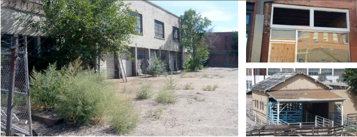
When reconstructing an element is impossible, develop a new design that is a compatible interpretation of it.
